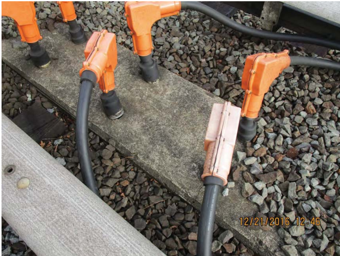
FIGURE 9 - OZ BUSHING COMPROMISED ON STUB-UP AND NEEDS REPLACEMENT f
