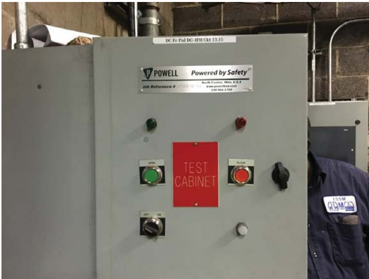
Figure 7 – POWELL BREAKER TEST CABINET
