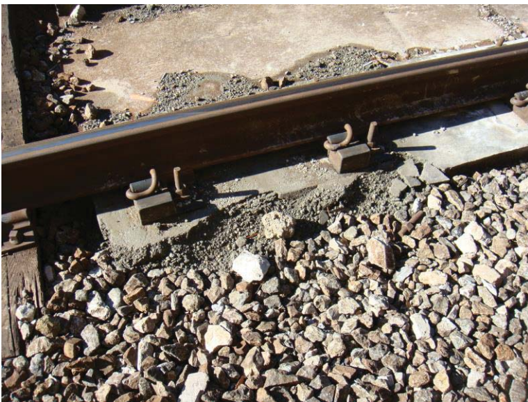
Figure 4 - B1 CM189+90 - Concern about concrete mix on new grout pad
