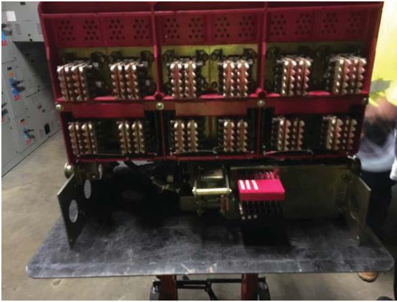
FIGURE 3 – POSTERIOR OF SECONDARY MAIN BREAKER, COPPER BUS STABS
