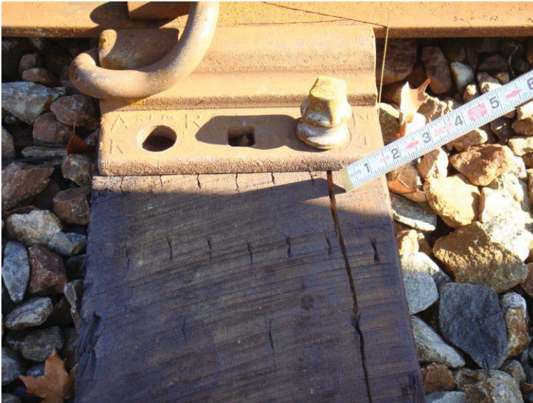
Figure 3 - Same tie - close up of split on right rail
