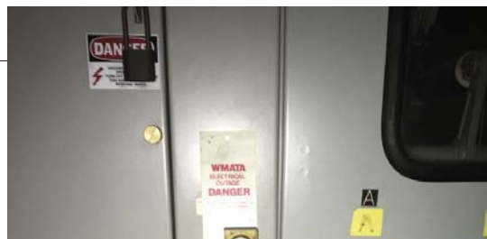
FIGURE 2 – LOCKOUT/RED TAG TO DE-ENERGIZE POWER EQUIPMENT
