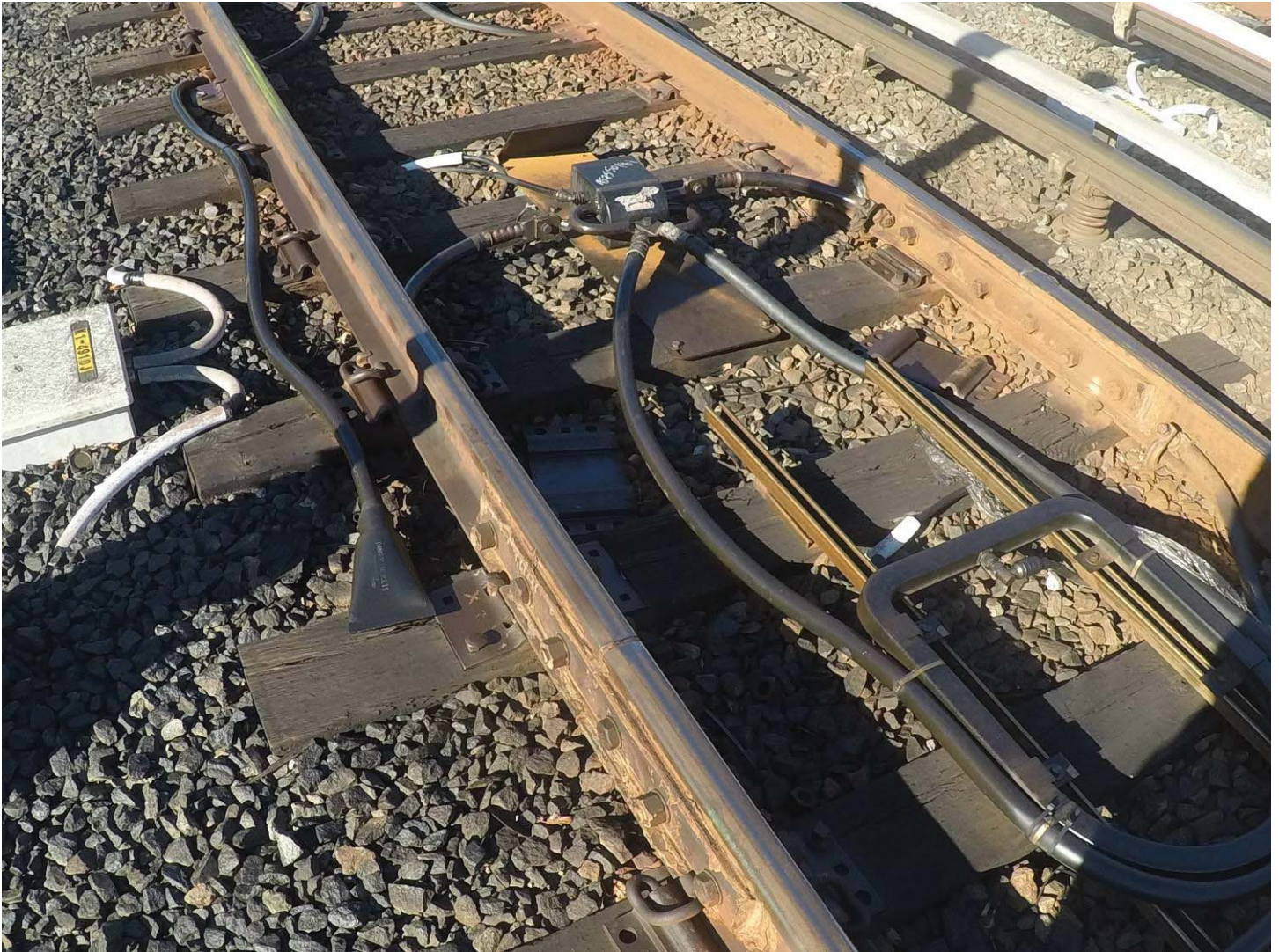
ATC cables booted at K1 491+00
