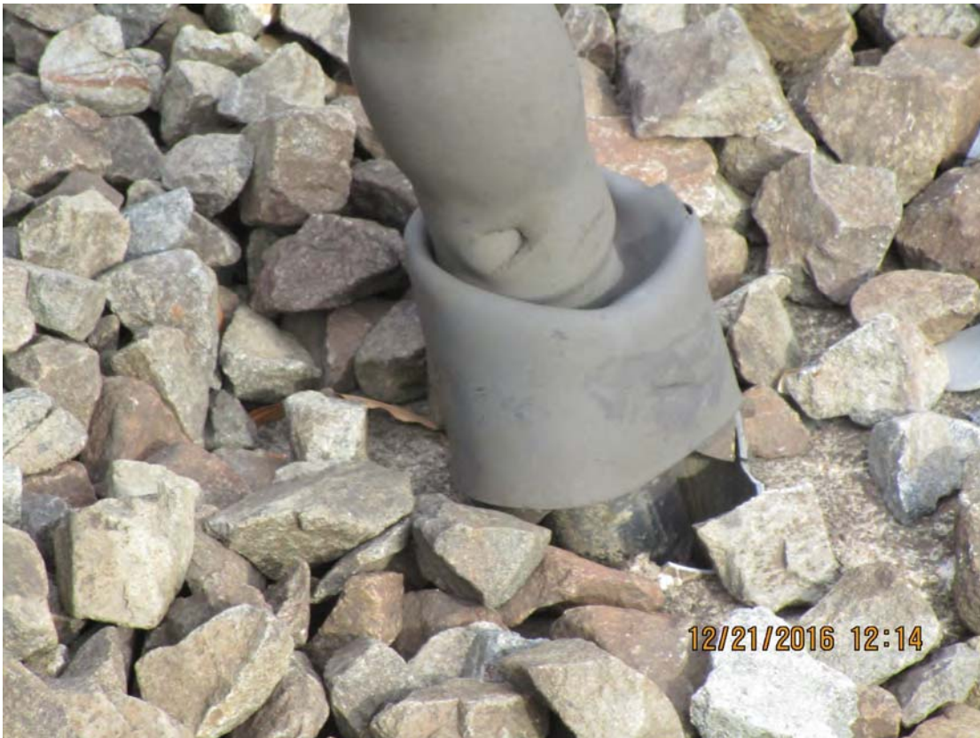
FIGURE 5 - STUB-UP CONDUIT COMPROMISED ON FEEDER CABLE TO 3 RD RAfL, BROKEN ORANGE BOOT Tf AT NEEDS TO f BE REPLACED, AND 3 RD RAfL COVER BOARD NEEDS REPLACEMENT f
