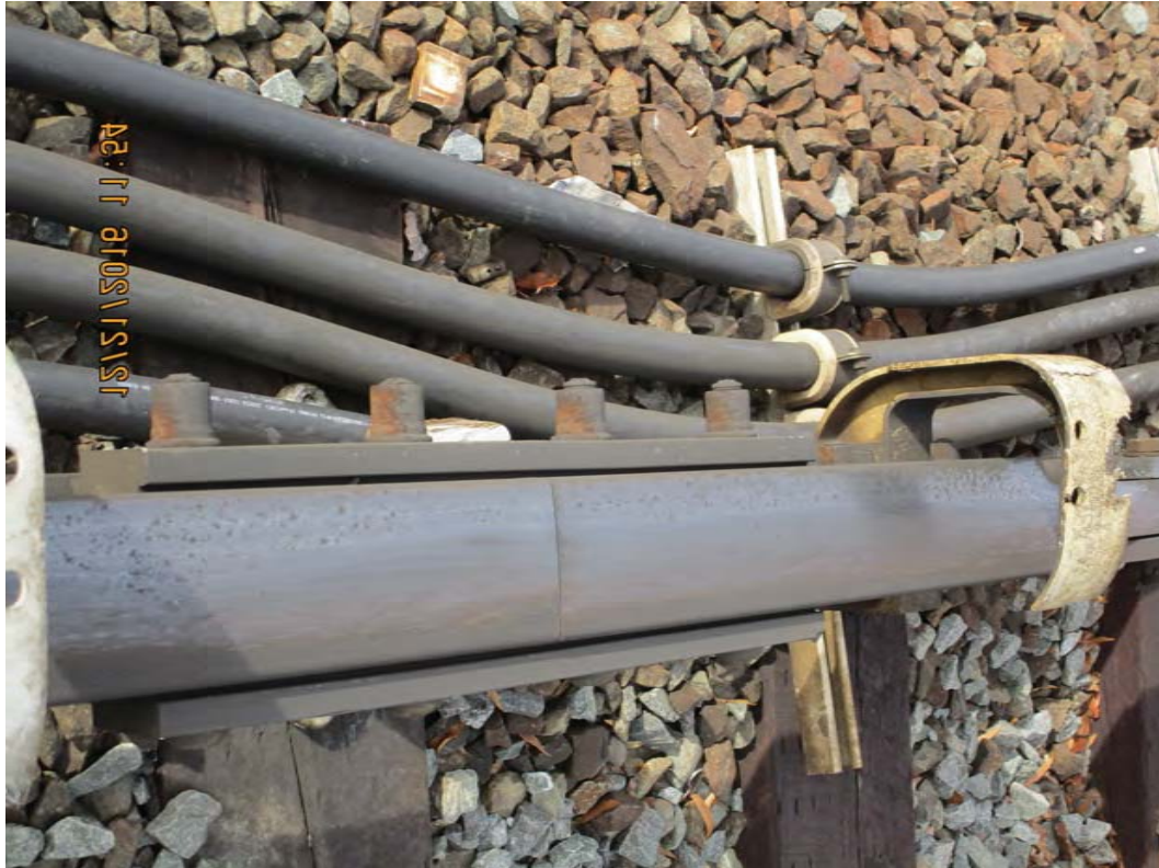
FIGURE 2 - CABLES LAYfNG ON DECK (BALLAST) AND 3 RD RAfL COVERBOARD BROKEN AND NEEDS f TO BE REPLACED f
