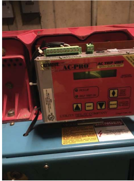
FIGURE 4 – TEST APPARATUS FOR SECONDARY MAIN BREAKER
