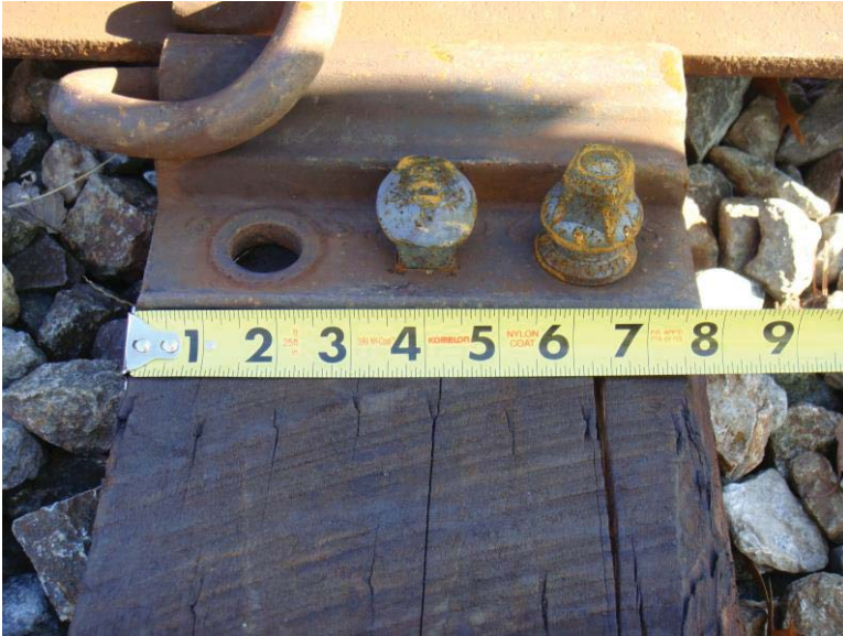
Figure 1 - B1 CM274+60 - 7 3/4" Crosstie - note split in line with fastener
