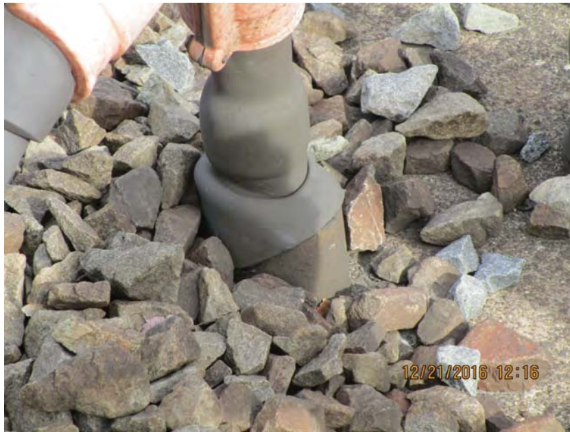
FIGURE 6 - BROKEN ORANGE BOOT, f EAT SF RfNK NEEDS REPLACEMENT ON STUB-UP TRANSITION FROM CONDUIT TO f ORANGE BOOT f
