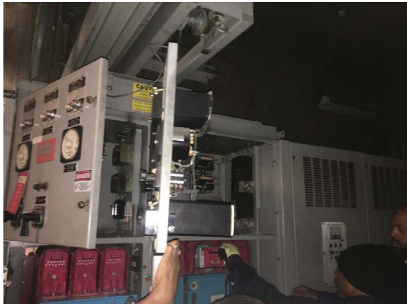
FIGURE 6 – SECONDARY MAIN BREAKER CUBICLE ON AC SWGR, TRYING TO TROUBLESHOOT THE RELAYS
