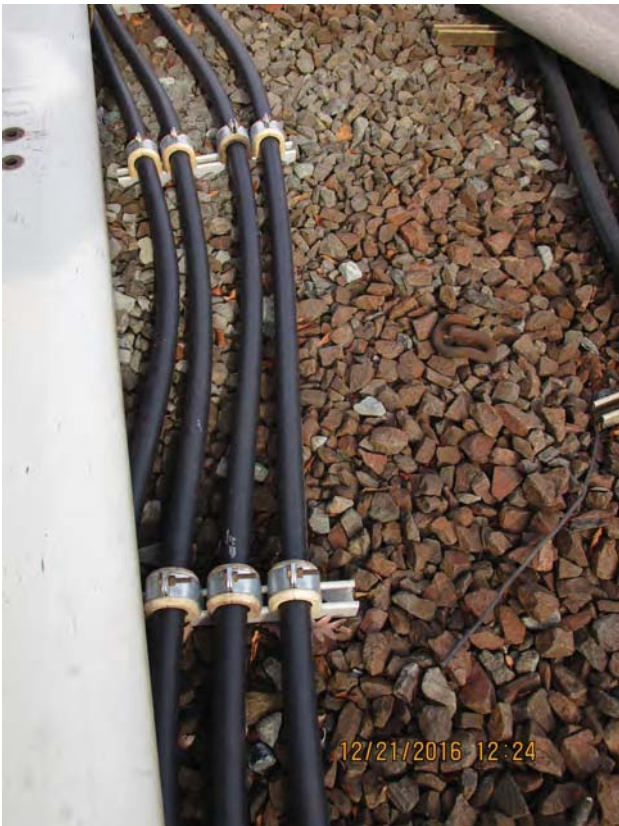
f FIGURE 7 - CABLES LAYING ON DECK (BALLAST), 3 RD RAFL COVERBOARD FALLEN OFF f
