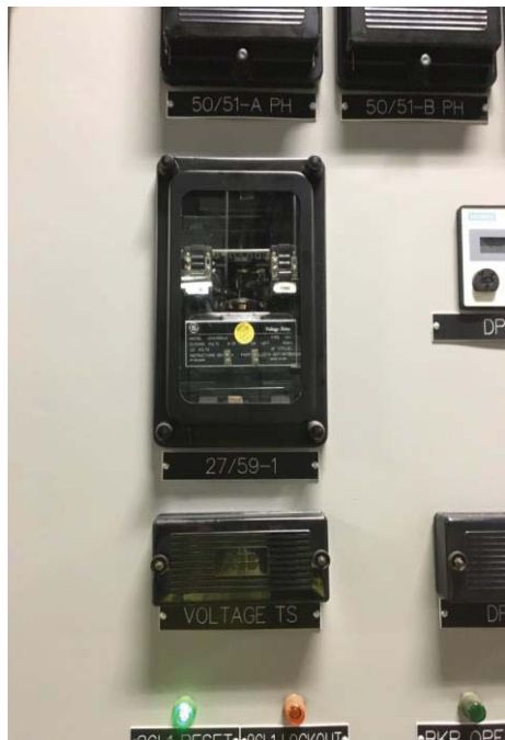
FIGURE 3 - GE UNDER/OVER VOLTAGE (27/59) RELAY
