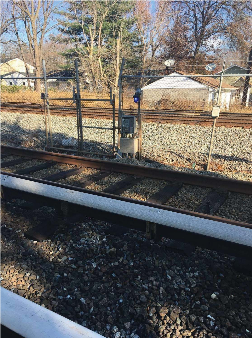
ETS Box with door missing A2 747+00
