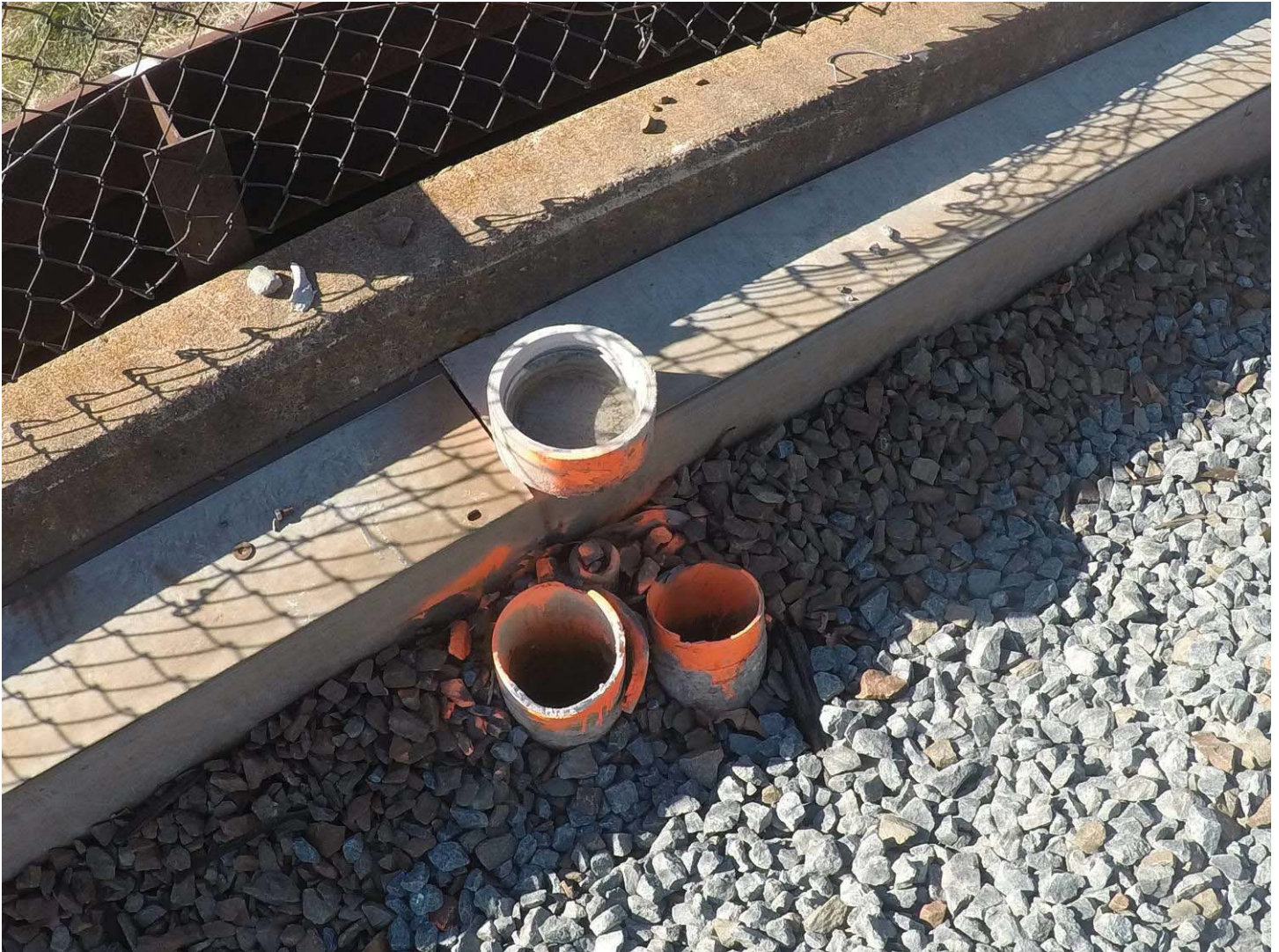
Damage to drainage access, marked for repair
