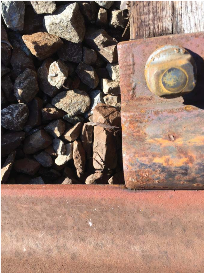
Figure 1 - Plate overhanging tie by one inch.
