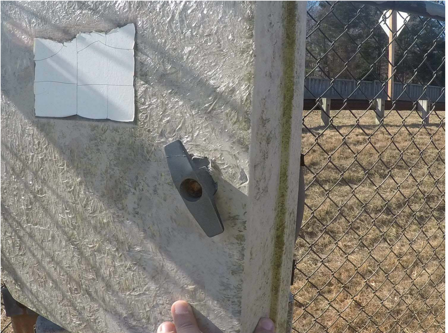
ETS Box with Broken Door Latch at K1 451+50
