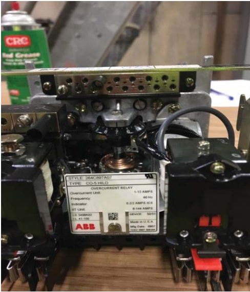
FIGURE 1 - ABB CO-5 HILO OVERCURRENT (50/51) RELAY
